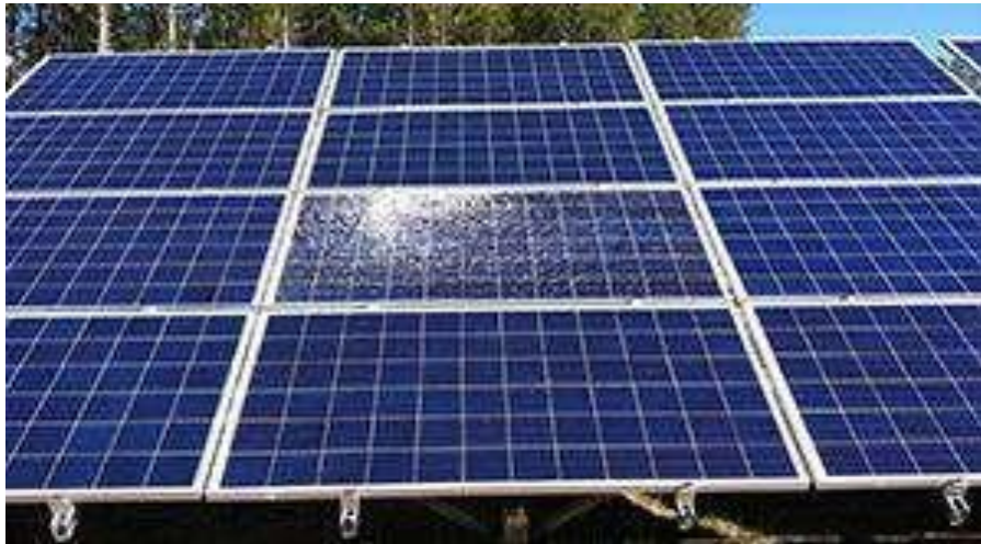
Fig. 10.2.3 Broken module in a PV array
