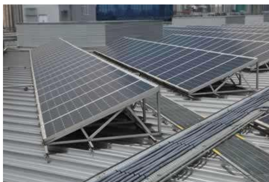
Fig. 10.2.16 Array mounting hardware to be checked
