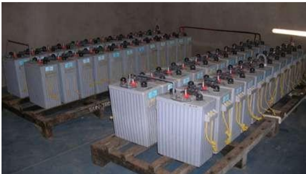
Fig. 9.2.5 Location of batteries in a well ventilated room
