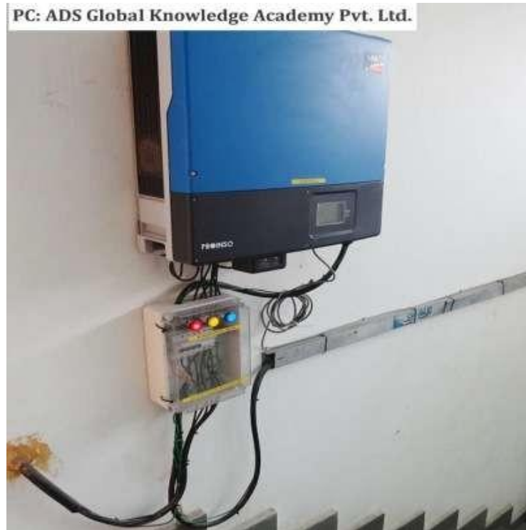
Fig. 8.5.7 Inverter and AC distribution box
