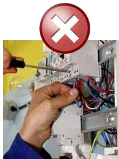
Fig. 11.2.6 Wrong way: Use of bare hands
