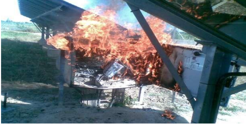
Fig. 9.3.6 Fire breaking out at the site of a solar PV system
