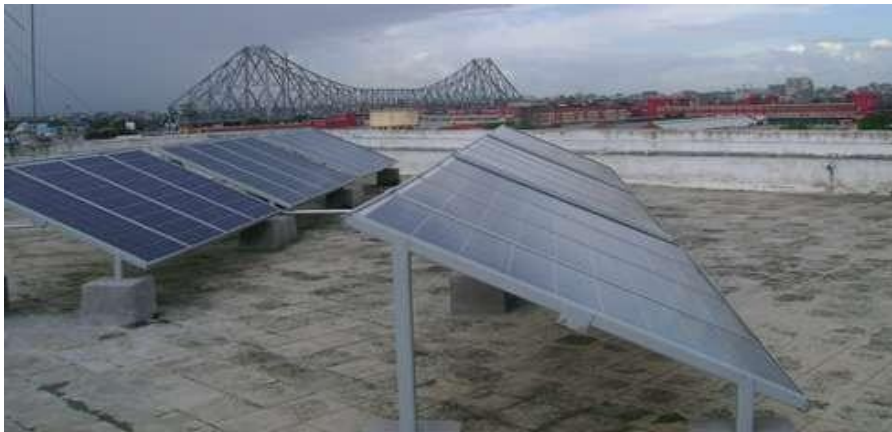
Fig. 9.2.1 Shadow free installation on Howrah Municipal Corporation Building
