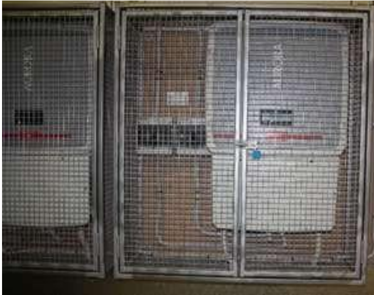
Fig. 9.2.3 Access to inverter is controlled
