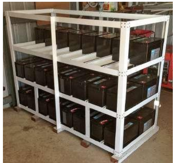
Fig. 8.5.1 Battery Bank enclosures/racks
