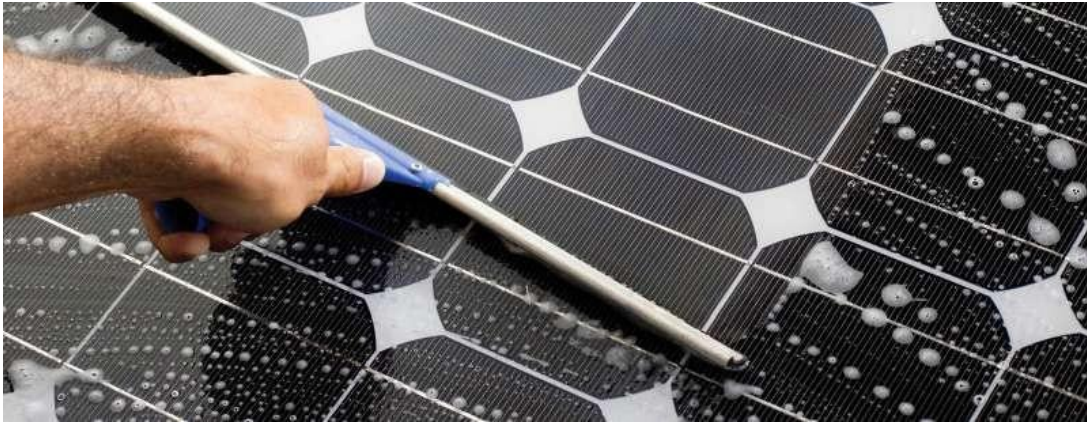
Fig. 10.2.1 Cleaning of modules using a wiper
