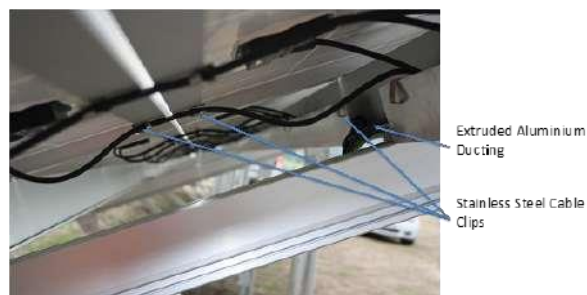
Fig. 9.3.2 Properly managed PV array cable
