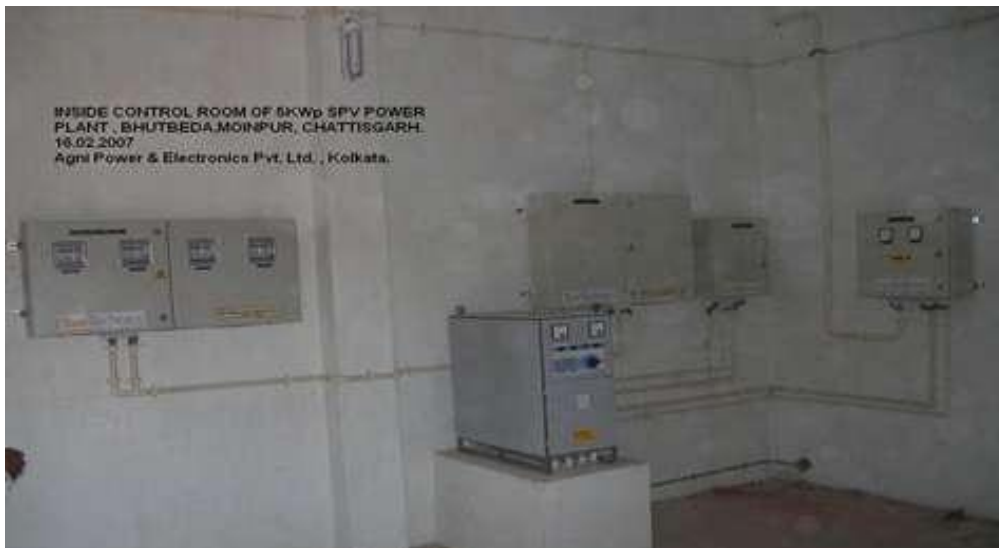
Fig. 9.2.4 Inverter and control equipment installed in a control room
