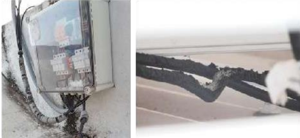
Fig. 9.3.3 Poor quality conduit and unprotected cable can be easily damaged
