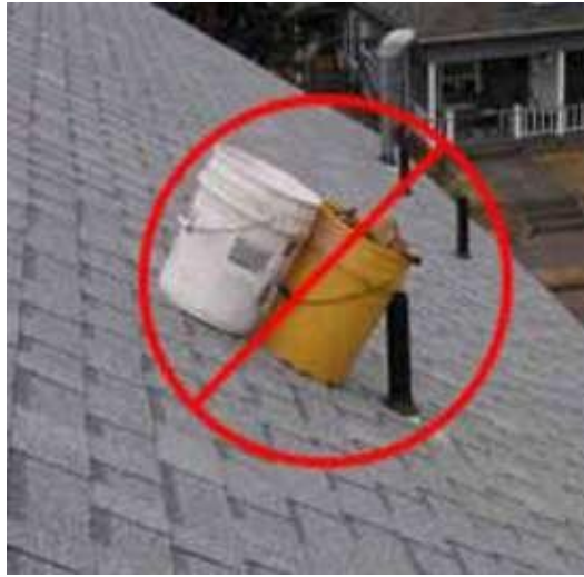
Fig. 11.4.4 Improper Placement of Tools
