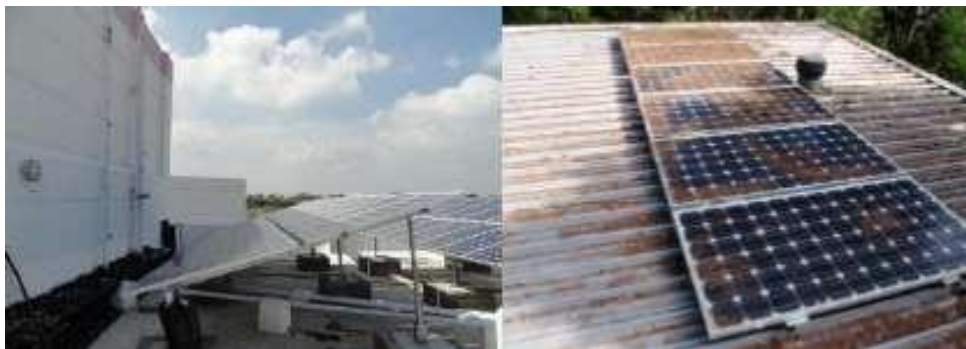
Fig. 9.2.2 Incorrect site selection for array installation
