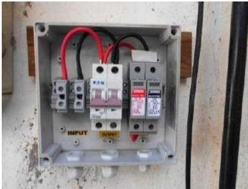
Fig. 8.3.6 AC distribution box (AC MCB for AC isolation, Surge protection device and Input side fuse protection)
