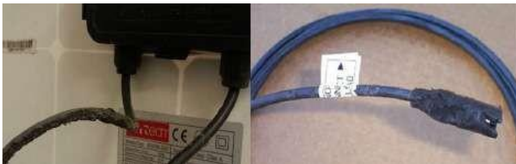
Fig. 10.2.15 Physically damaged wires
